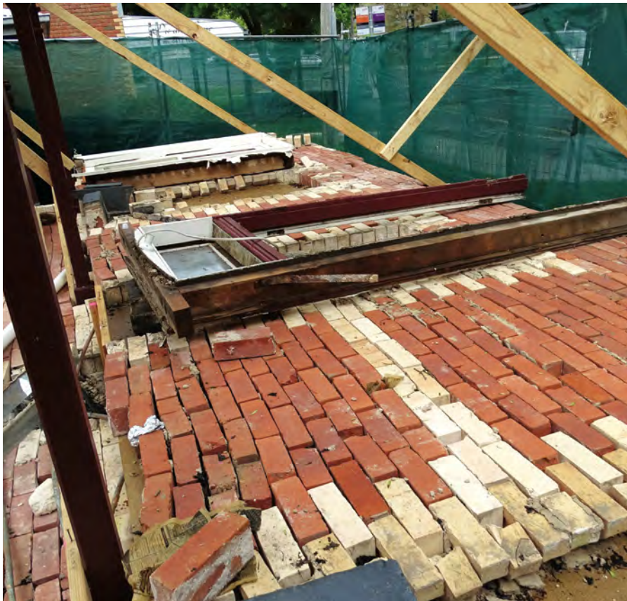
Left: In the early stages, each brick from the cottage's façade was removed, numbered and laid in order. Below: Award from the National Trust.
