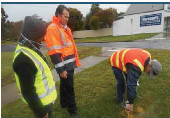
(L to R) Council Project Manager Mukal Hatwell, and Signage Manager Alan Jones watch Russell Anderson mark the location for one of the new signs on Warrenheip Street.
