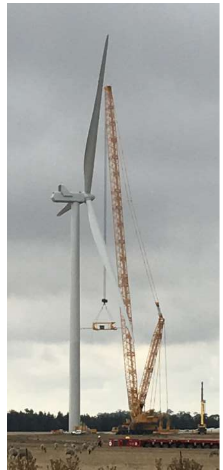
Photo shows turbines at Lal Lal Windfarm in various stages of construction while the new power pole in the foreground carries the three 30mm thick power cables (lower bank of 3) that will supply power to the grid at the Ballarat Area Terminal Station.
