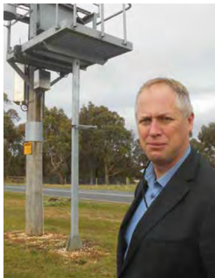
Powercor's Richard Scholton announcing the installation of the battery on the Durham Lead Road in August 2015.
