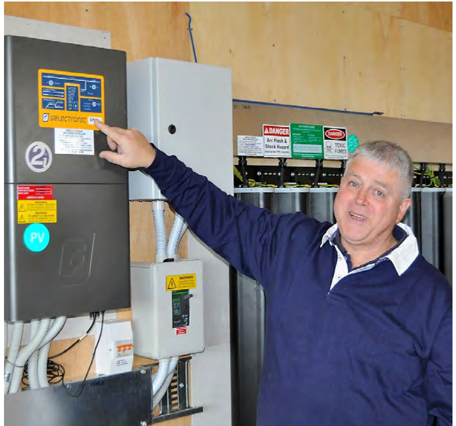
Peter Denniston in his workshop with the controls that regulate the house's energy production and usage. On the right is the battery storage array that, although expensive, is designed to last for thirty years.
